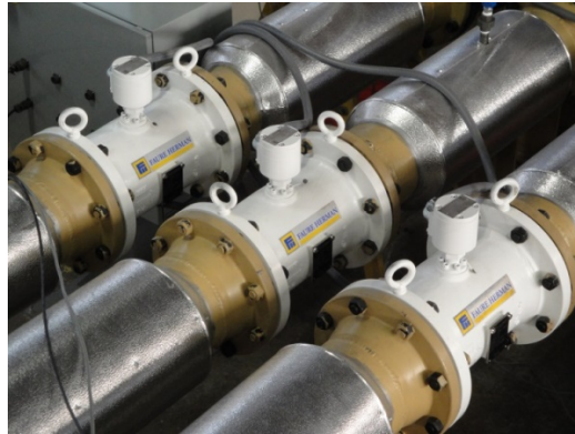
Fig. 11. 6" Liquid Turbines at the CEESI Oil Facility.
