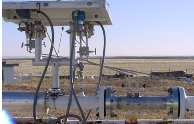
Fig 2. Water Flow calibrated Cone DP Meter Installed in a Gas Pipeline.
