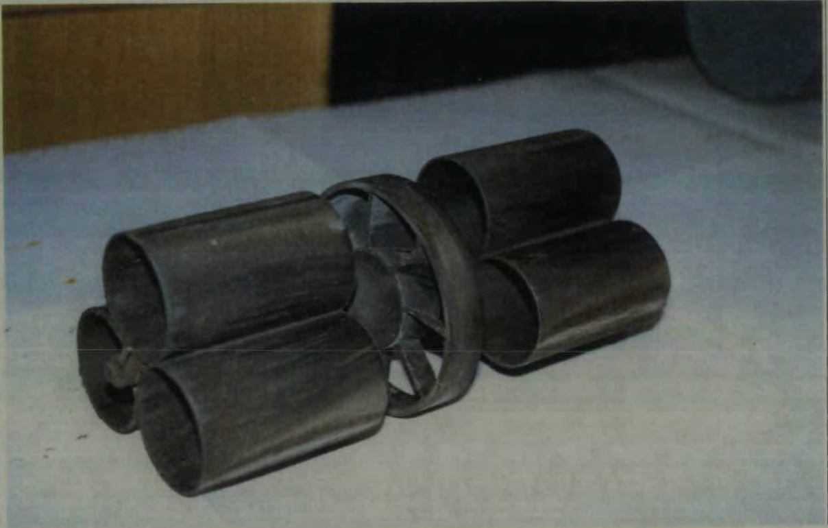
Figure 8. Scale deposits on internals of turbine meters.
