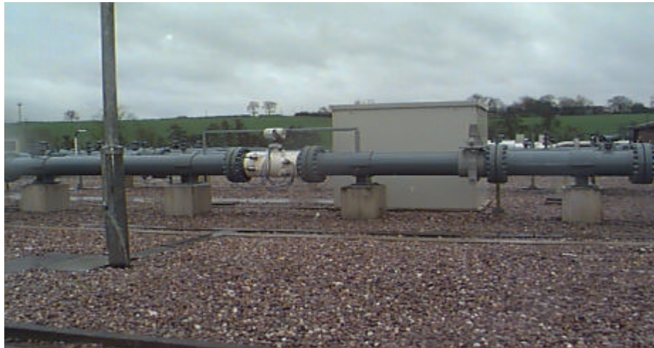
Figure 8 - USM and Orifice Plate Installation
