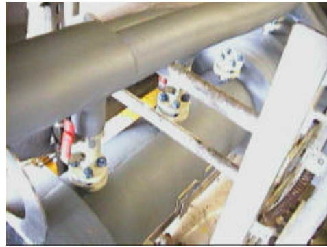
Fig. 20 - The Installed Trial Meter
