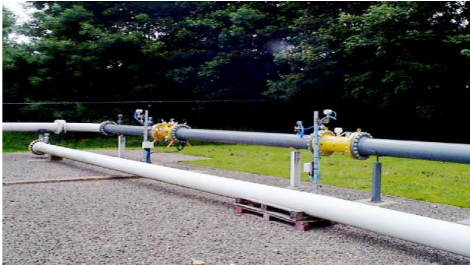
Figure 1 Ultrasonic Meter and Turbine Meter Installation
