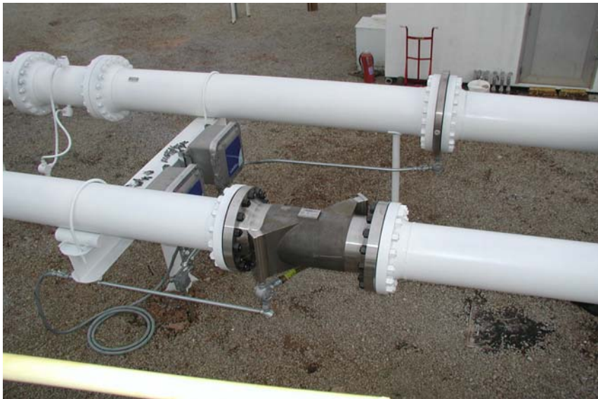
Figure 2: Installed LEFM 240C
