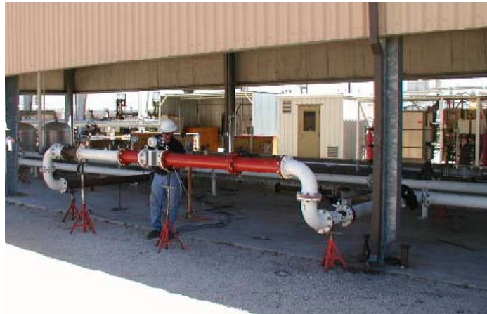
Fig. 15 – A tested 6"-meter installed 13D behind a double elbow out of plane
