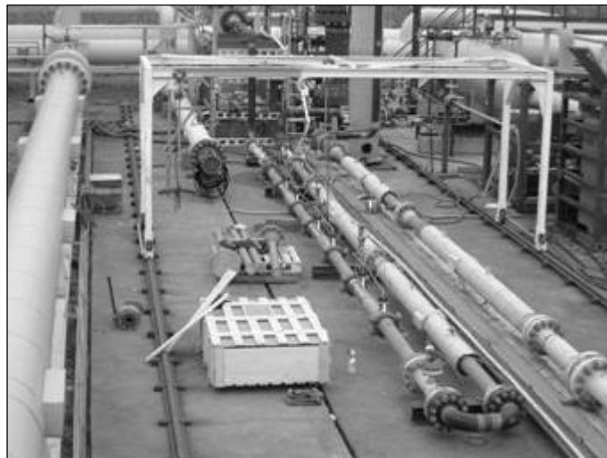
Figure 11. Overview of the K-Lab test site.
