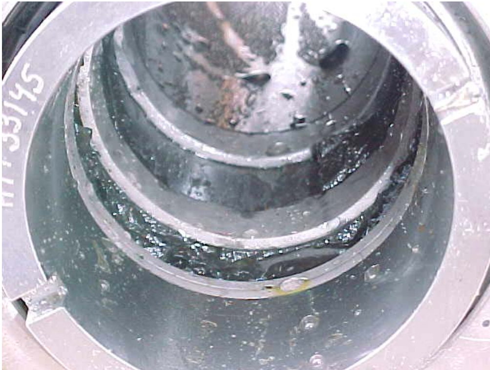
Figure 14. An inside view of MFI meter before repair in late 2002.
