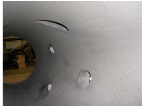
Figure 23 –Dirty 10-inch Meter
