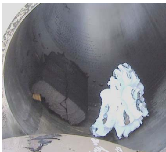
Figure 35 – 12-Inch Meter Blockage
