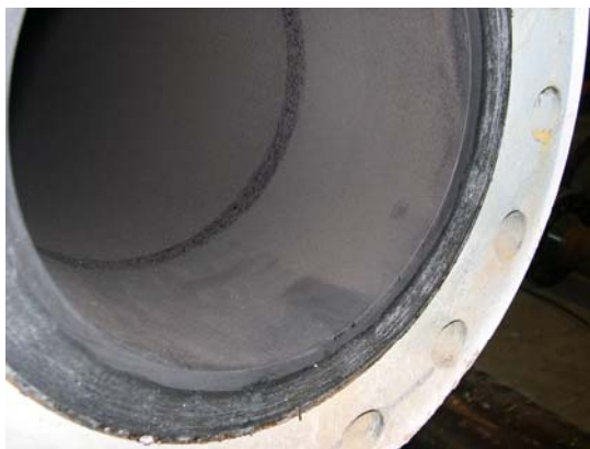
Figure 22 –Dirty Upstream Meter Tube
