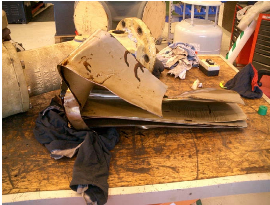
Figure 11. Defect flow straightener from GOHS line 4.
