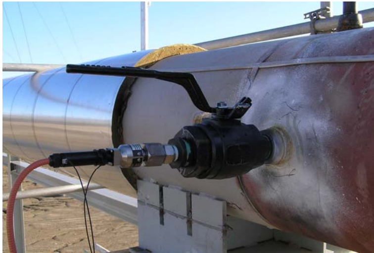
Figure 13. Insertion Focus™ Probe installed in a 12-inch pipe, gas processing plant, Alberta, Canada
