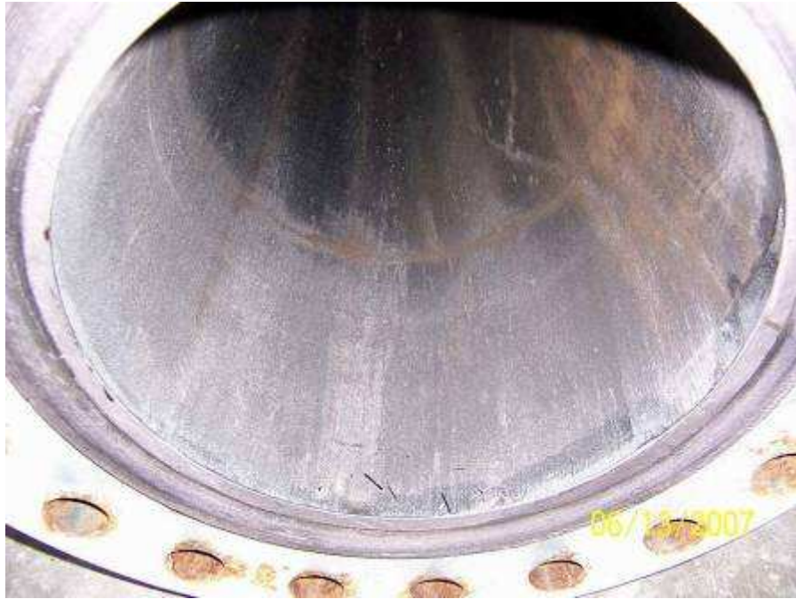
Figure 17: 12-inch Dirty Piping
