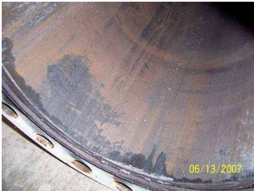
Figure 18: 12-inch Dirty Piping Close Up
