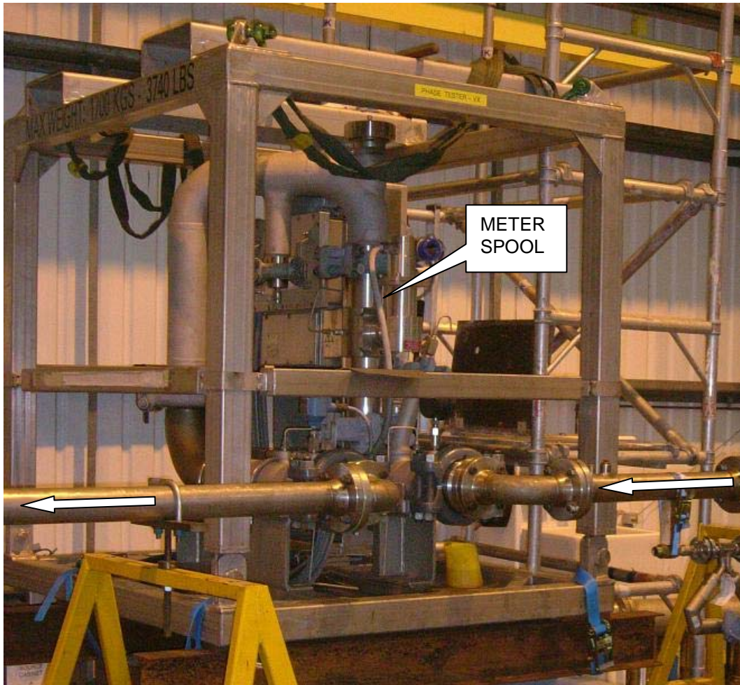
Fig. 19 – Vx meter skid installed in the TUV NEL Multiphase Test Facility (Scotland).
