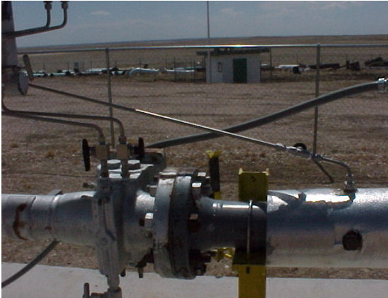
Fig 3. Orifice fitting with natural gas flow.
