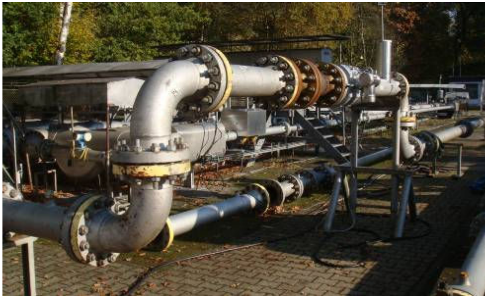
Figure 31: The V12 tested at 90° rotated with a double bend out of plane at 10D distance.
