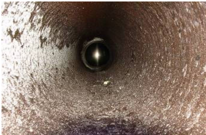
Figure 8, fouling evenly distributed over the pipe wall
