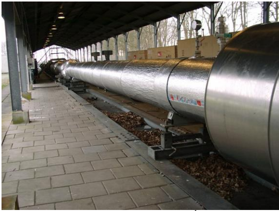
Figure 11 - Thermal lagging; Jan. 9 th 2009,
