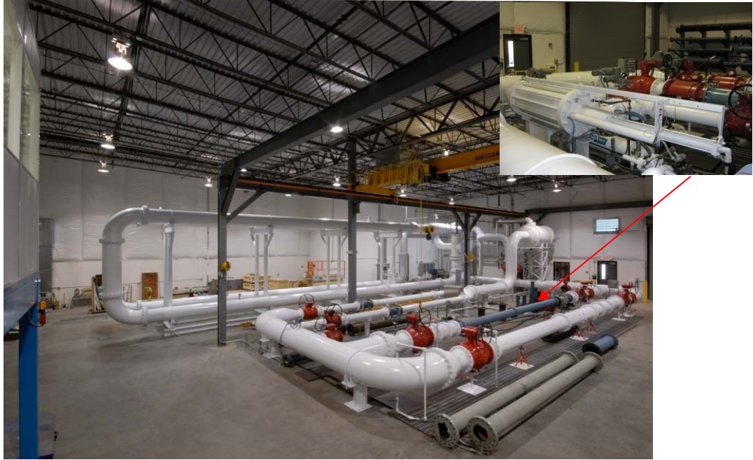
Figure 1 The Cameron calibration facilities
