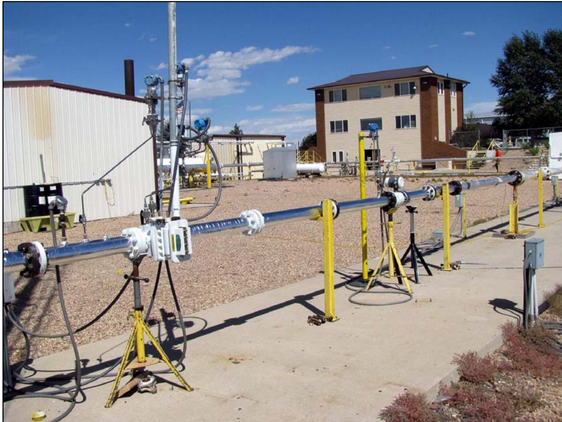
Figure 4 – 3-inch Orifice and USM Installation, August 2010
