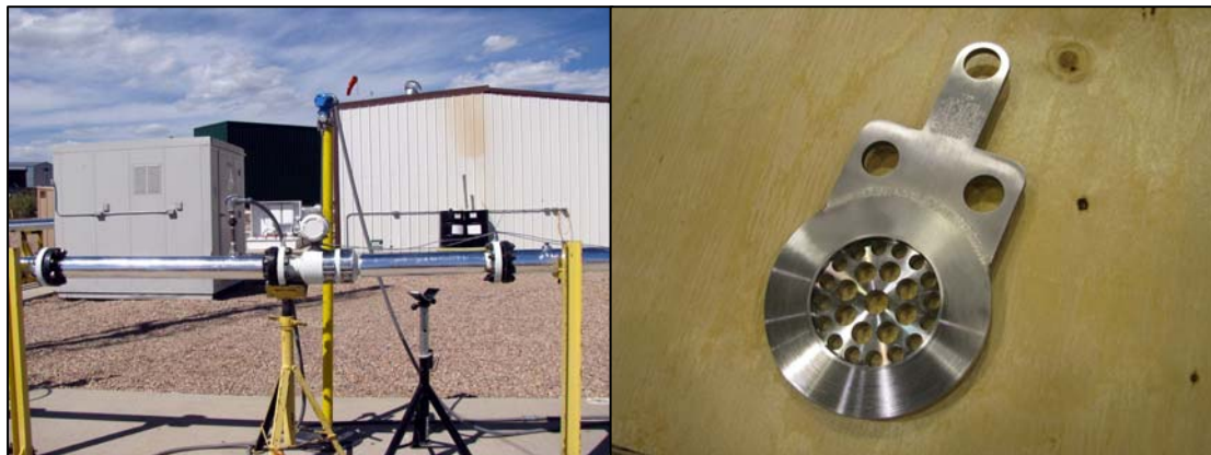
Figure 5 – 3-inch USM and Piping
