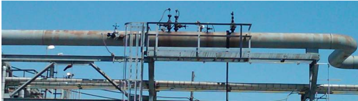
Fig. 29 24" flare line now with both original Bias 90 installation and with diametrical Diagonal 45 installation
