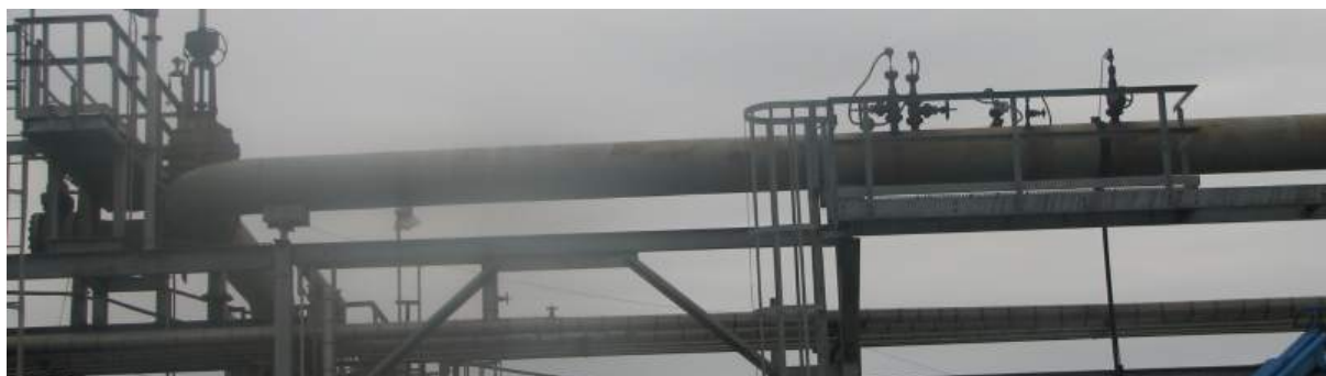
Fig 25 A 24" flare with a Bias 90 installation on the top of the pipe. Stratification and convection flow producing peaks of low flow based on the ambient temperature, but not evident at the flare tip.
