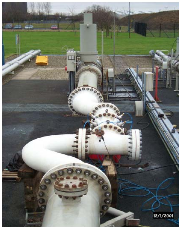
Figure 6. USM installed at test facility with OD upstream straight pipes
