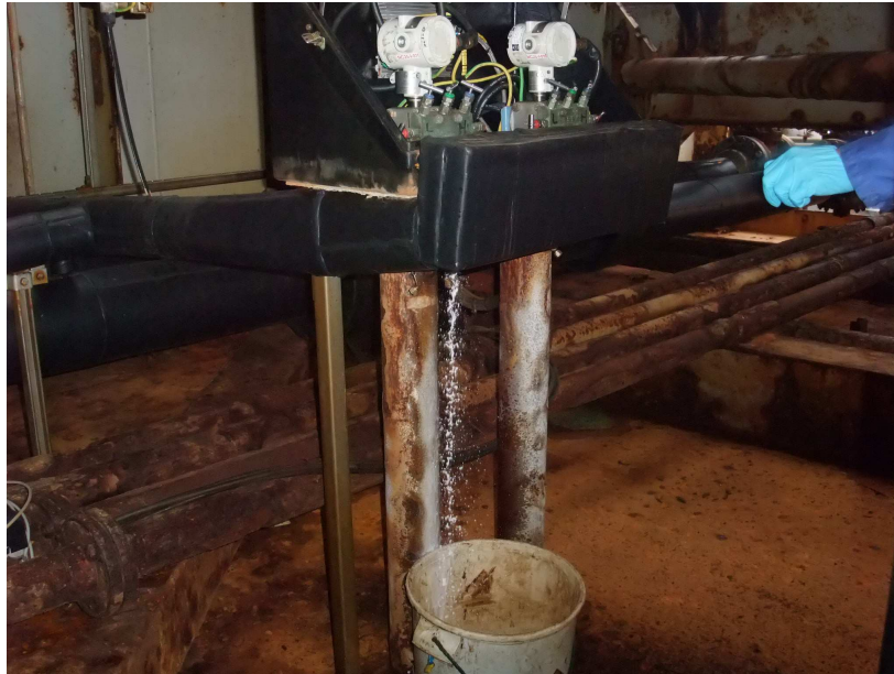
Figure 7:- The challenges of liquid build-up in gas metering streams – worst case scenario!
