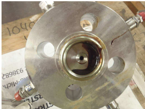
Figure 14:- Oil residue in pressure transmitter manifold
