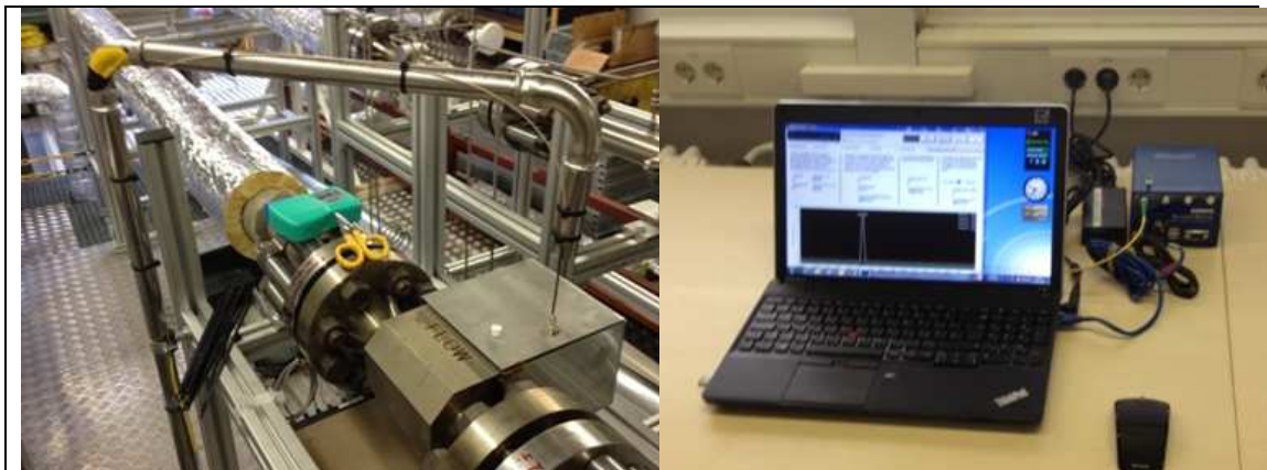
Figure 8: Photos of the fibre optic flow meter installed in the AREVA Benson test loop.
