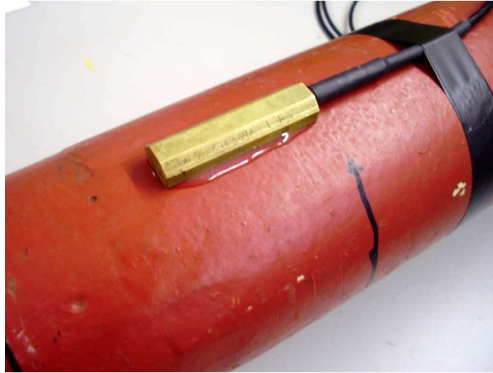
Fig. 16 – Standard National Grid Gas longitudinal surface sensor installed on a three inch pipe before applying insulation
