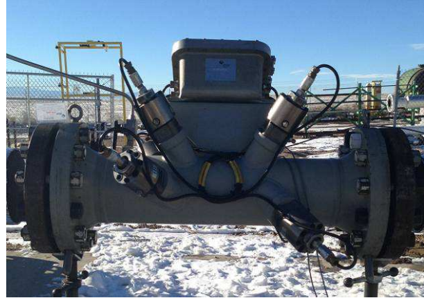
Fig 26. Integral Three Bounce Path Ultrasonic Under 8” Wet Gas Flow Tests at CEESI
