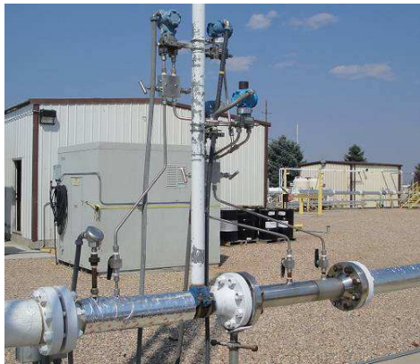
Fig 17. 4” Venturi Meter Two-Phase Wet Gas Flow Tests.
