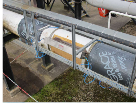
Figure 4 : Stream 1300 clamp on meter installation
