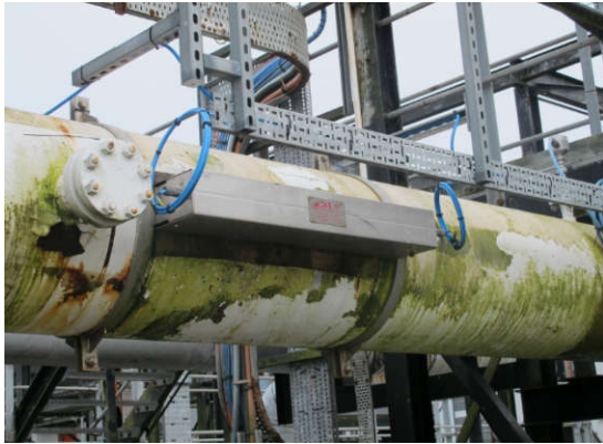
Figure 3 : Stream 1200 clamp on meter installation
