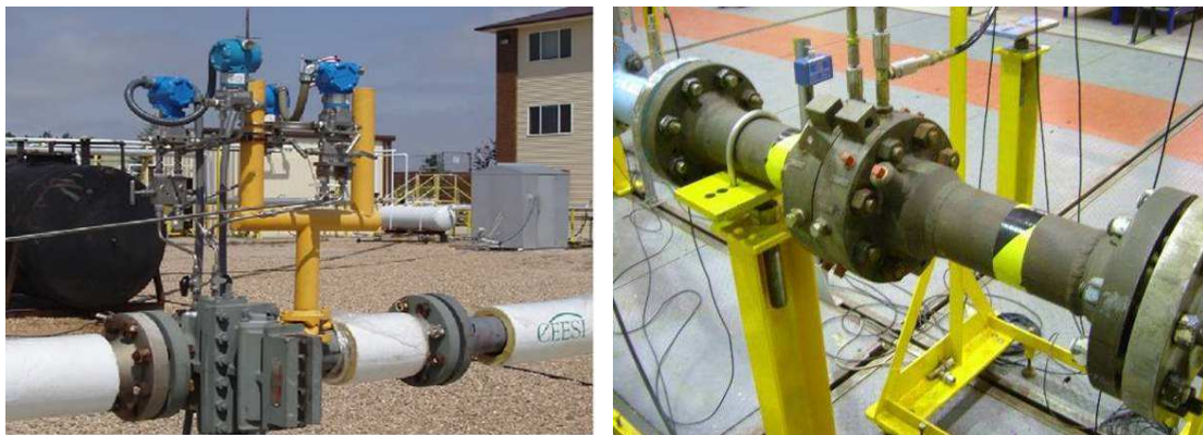
Fig. 1 - Orifice meter installed in CEESI Wet Gas Facility (left) and in NEL Wet Gas Facility (right).
