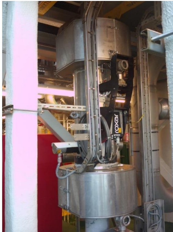
Figure 12: MPFM measuring Ivar Aasen import line at Edvard Grieg
