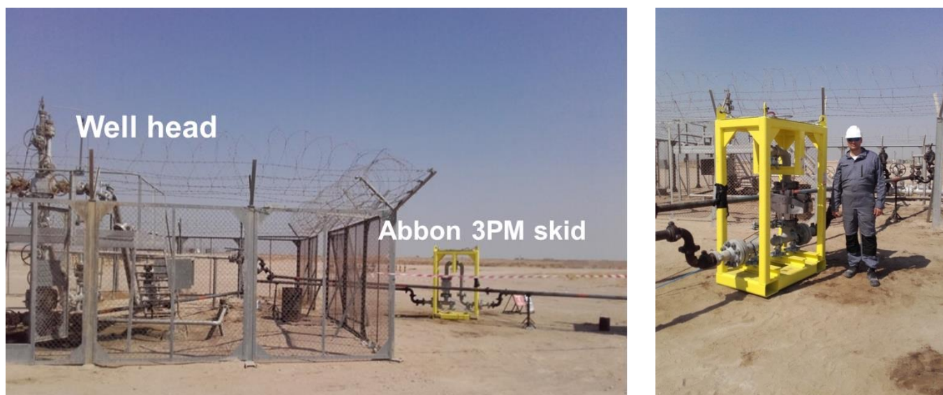
Figure 7 Abbon skid in mobile field application. Left: Connected to a wellhead and a mobile test separator, Right: Compact skid with Abbon's field supervisor
