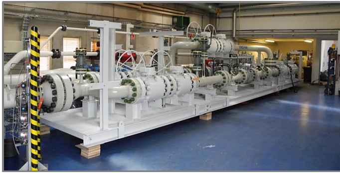
FIGURE 7 : SKID 1 AT THE CALIBRATION STATION OF FORCE TECHNOLOGIES
