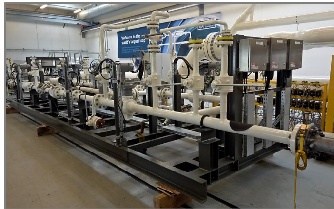
FIGURE 21 : SKID 3 AT THE CALIBRATION STATION OF FORCE TECHNOLOGIES
