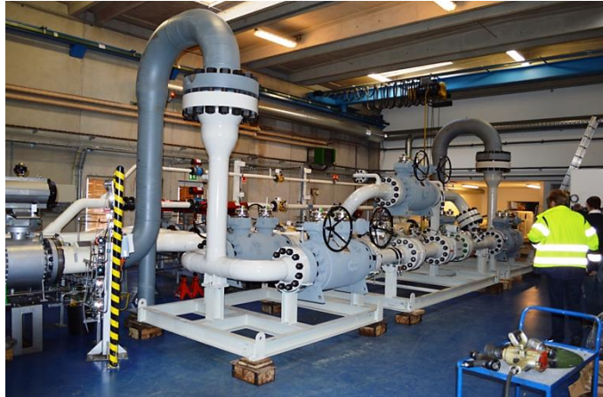
FIGURE 15 : SKID 2 AT THE CALIBRATION STATION OF FORCE TECHNOLOGIES
