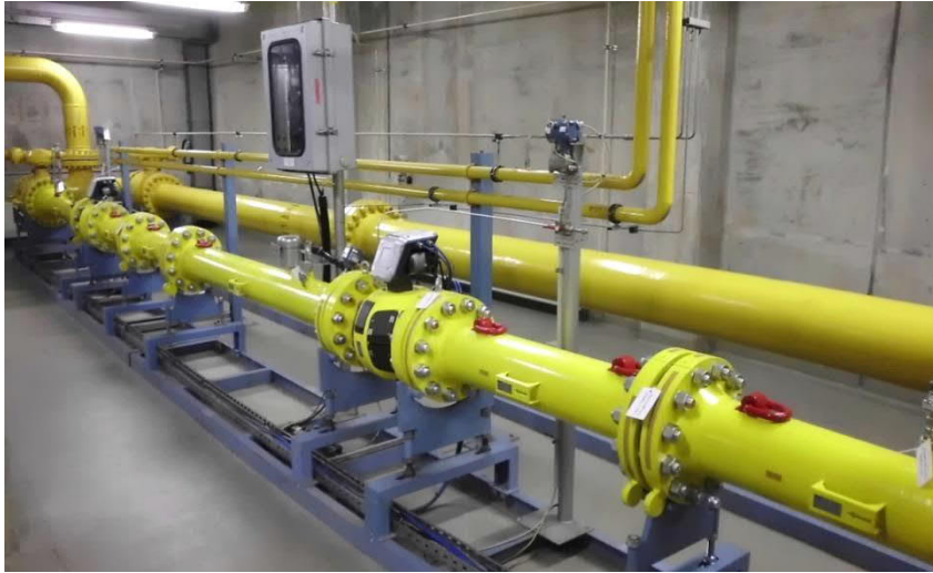
Figure 6: Serial installation of two USMs, metering station B
