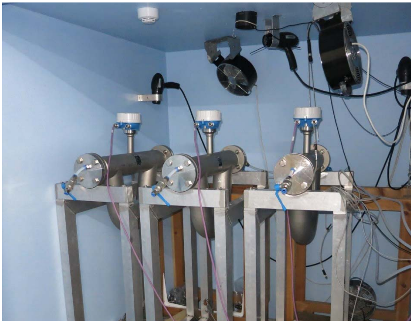
Figure 4: Test installation of three Promass Q DN50 in H&D Fitzgerald's temperature-controlled chamber [2].
