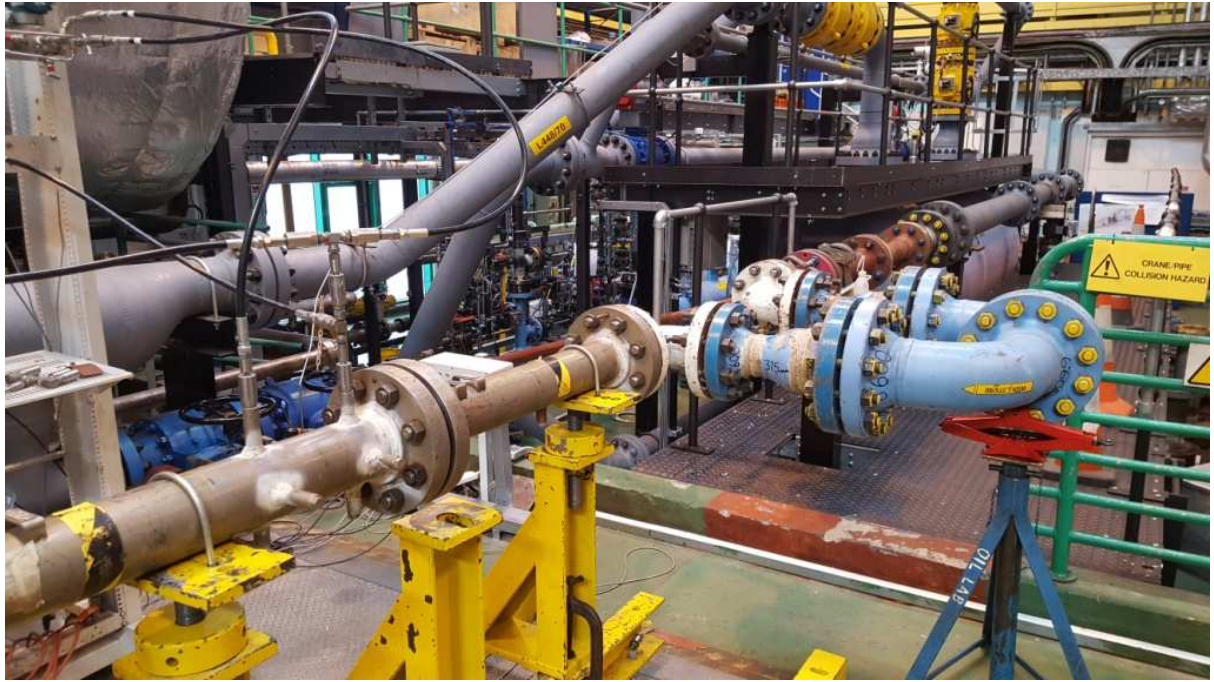
Figure 1 Photograph of the installation effects test. The bend combination is 10D upstream of the Venturi tube.
