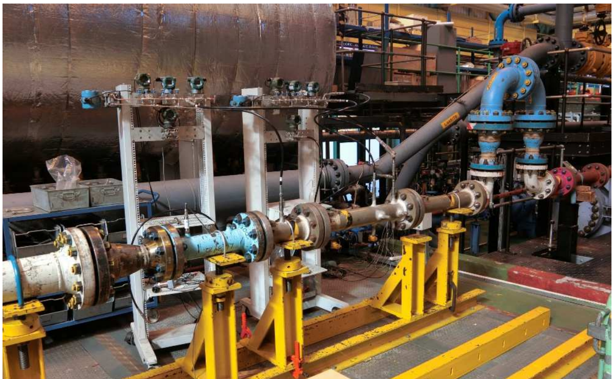
Figure 2 Photograph of the installation effects test. The bend combination is 10D upstream of the Venturi tube.
