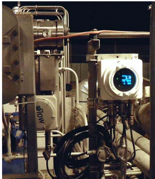
Figure 1: Field Installed Microwave Water Cut Meter
