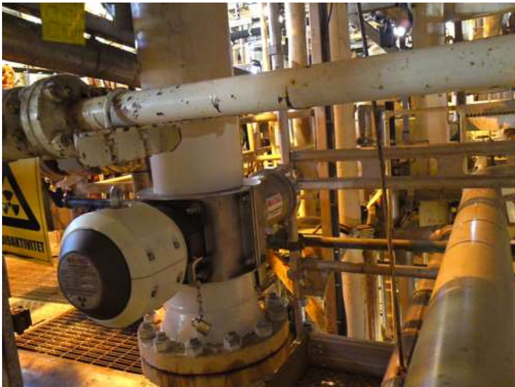
Figure 3 DT on process pipe
