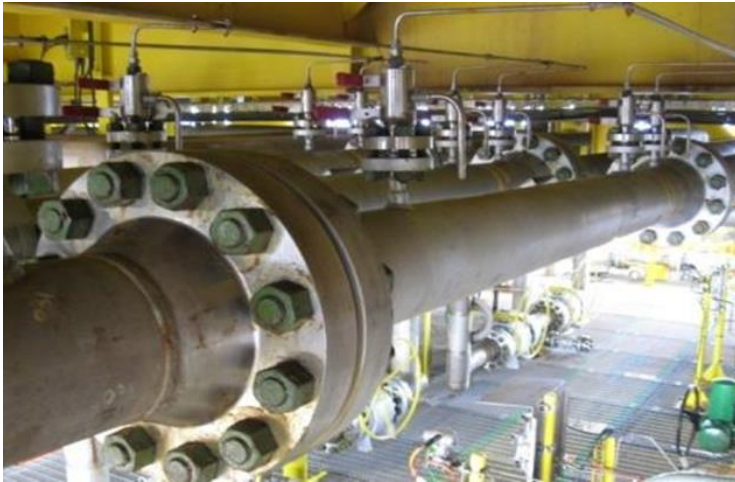
Figure 1. Bank of WGMs for wellstream monitoring
