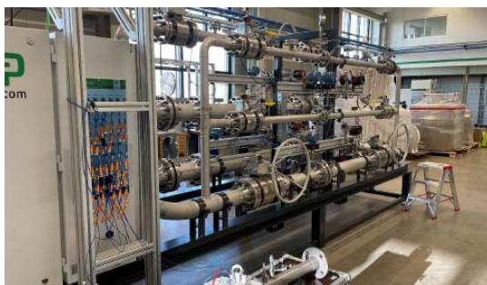
Figure 5: Skid with nozzles
