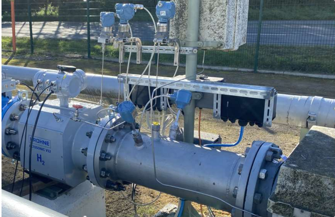
Figure 6: The 10" ALTOSONIC V12 (150#) ultrasonic flowmeter installed on site.
