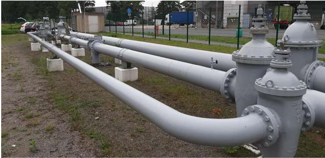
Figure 2: Hydrogen pipeline at industry park Marl.
