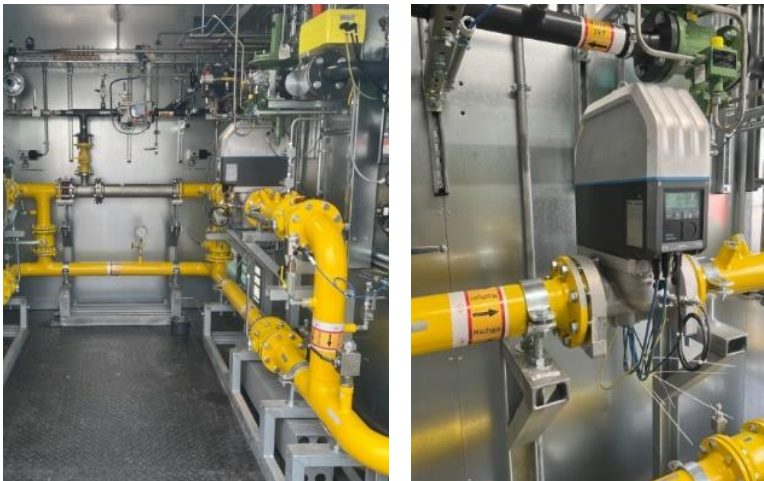
Figure 3 FLOWSIC500 in the mixing station of the avacon pilot project "Hydrogen in the gas network"
