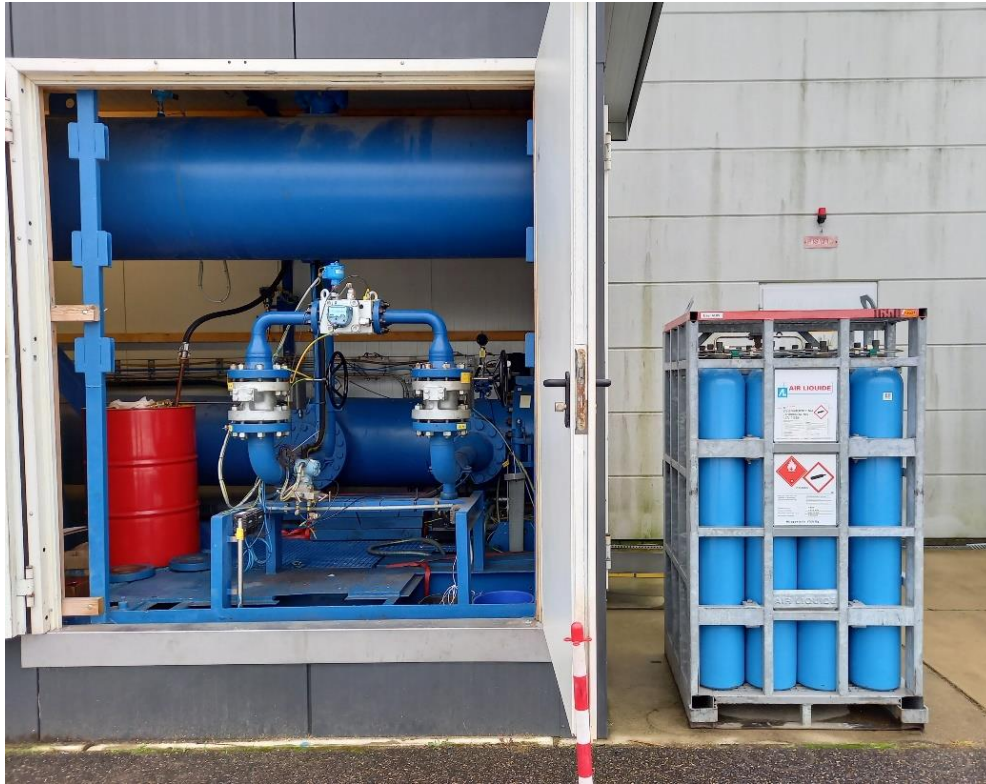
Fig. 1 – MuT mounted on VSL’s GOPP, accompanied by hydrogen gas cylinders.
