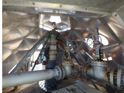
Fig 6. Inside Well Head Enclosure.
