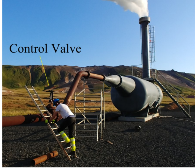
Fig 14. Flow Control Valve Upstream of Separator.
