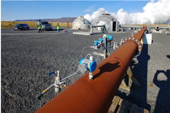
Fig 5. Orifice Meter Downstream of Well Head.
