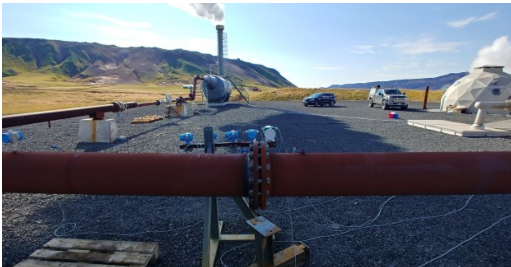
Fig 9. Orifice Meter Under Test with Saturated Steam Separator Downstream.
