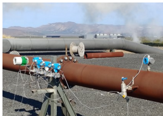
Fig 2. Orifice Meter Saturated Steam Flow Test.
