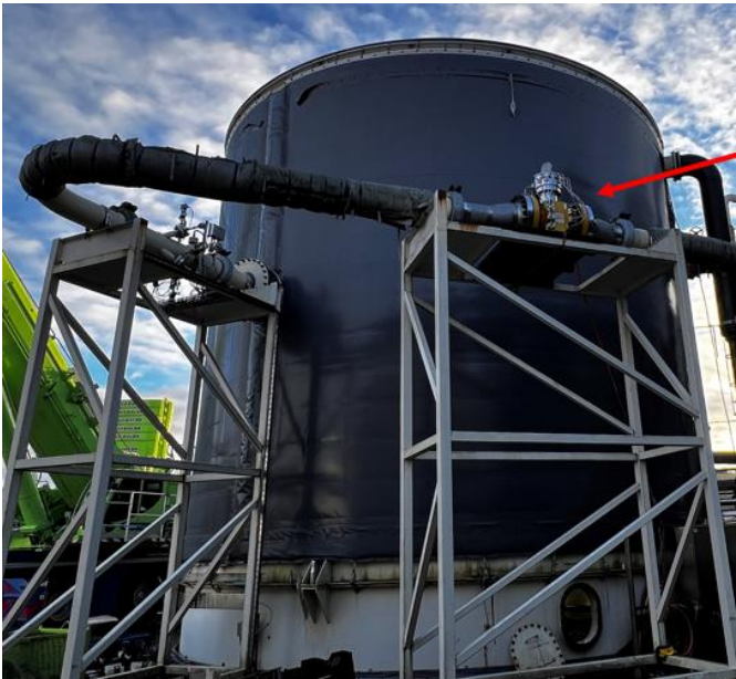
Figure 8 Location of the test meter outside the water tank where the compressors are submerged. Note the long horizontal pipe upstream the meter.
