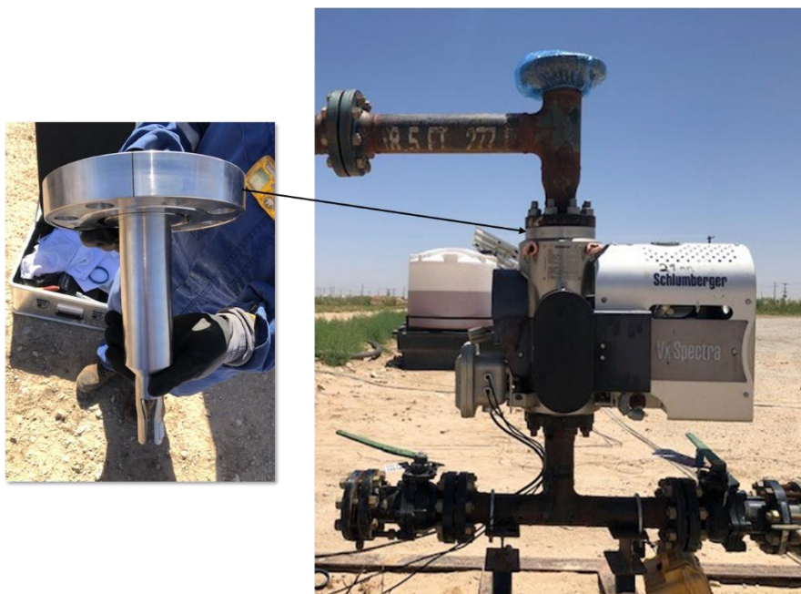
Figure 13 – Typical installation of MPFM equipped with XRF source and LRE in the Permian basin, Texas, US.
